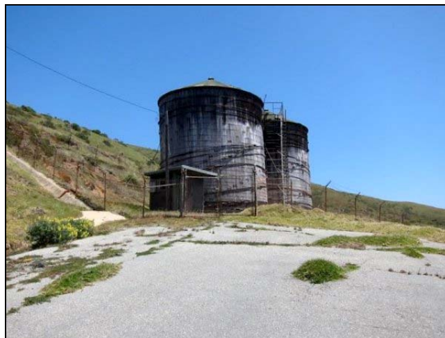
Figure 11. Redwood water storage tanks on the hillside parcel east Highway One.
